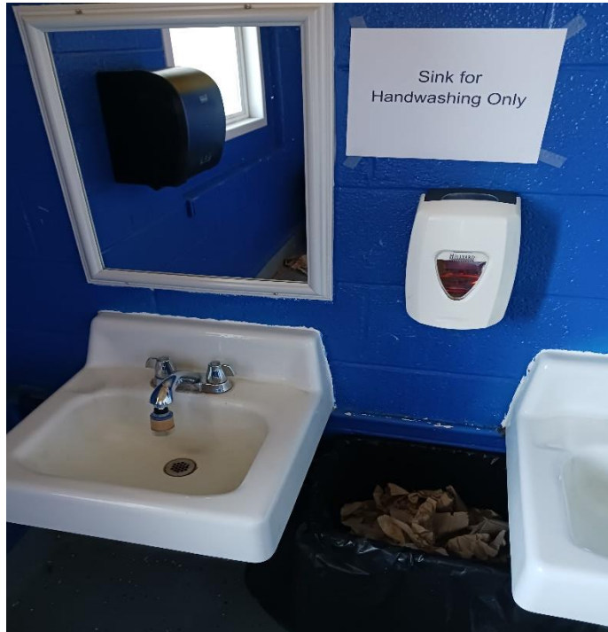
Signage placed adjacent to 164-MTS-12 and 164-MTS-13
